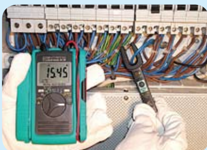
Measuring current in a Switchboard
